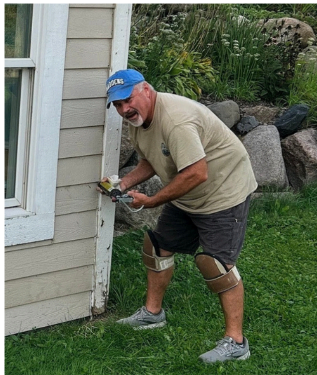
Andy Turner wields a mean caulk gun to patch up a corner of the farm house.
