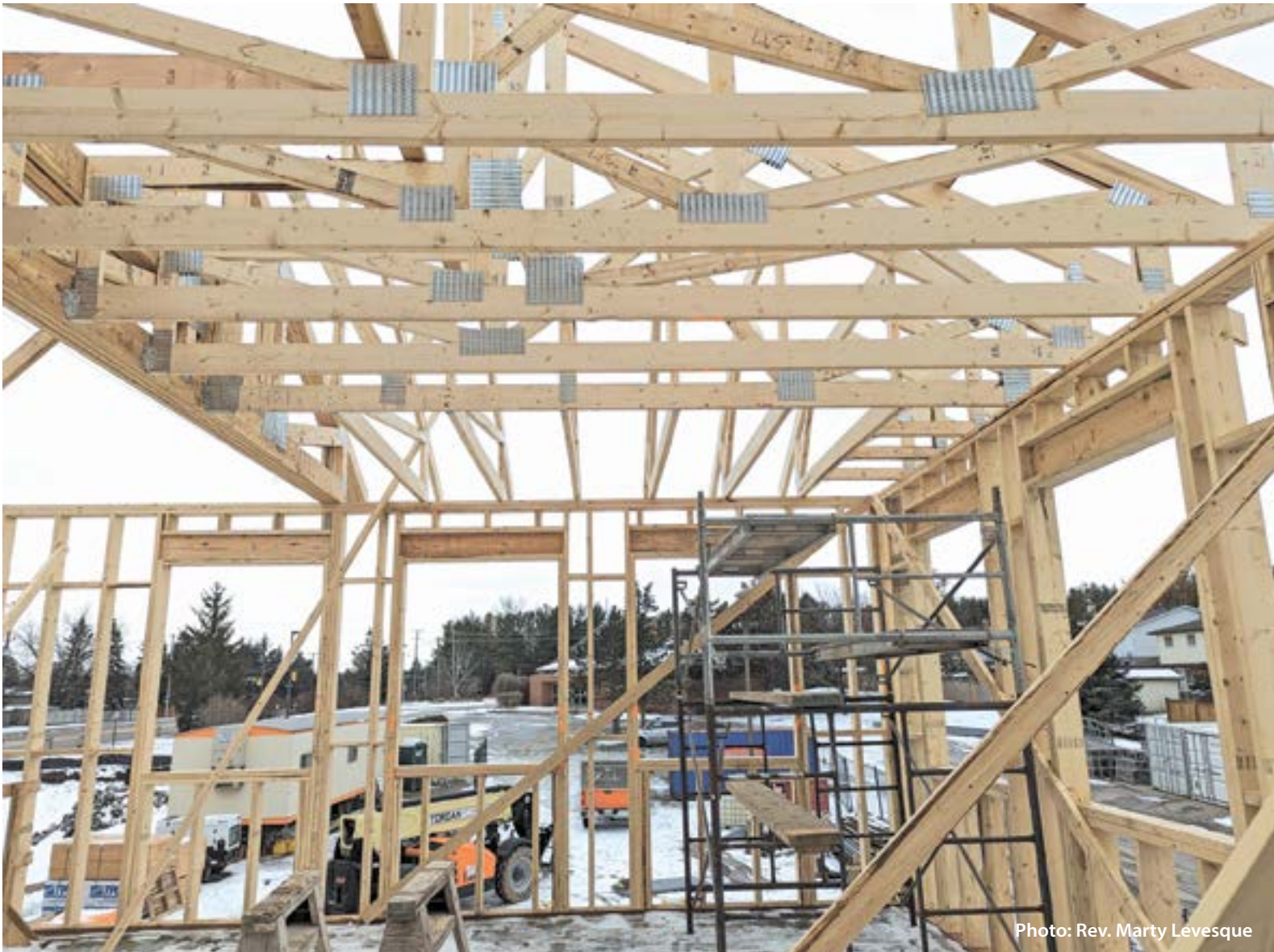
Building a new church: Not an everyday sight in the diocese. (All Saints', Waterloo, January 2023)
