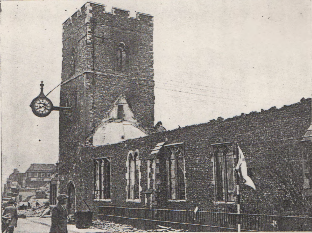
St. George's Church, with roof gone and tower unsafe, flew the flag of St. George from a post on the pavement. The clock records the time, 2,20.
