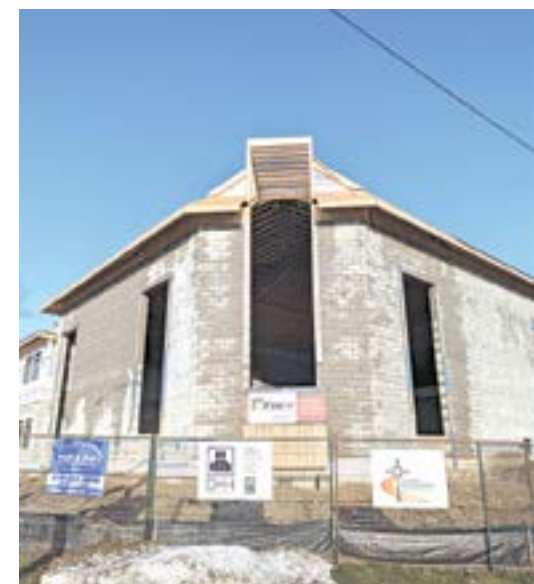
From the ground to the highest point translucent glass will be accentuated with a large cross that will be illuminated at night.
