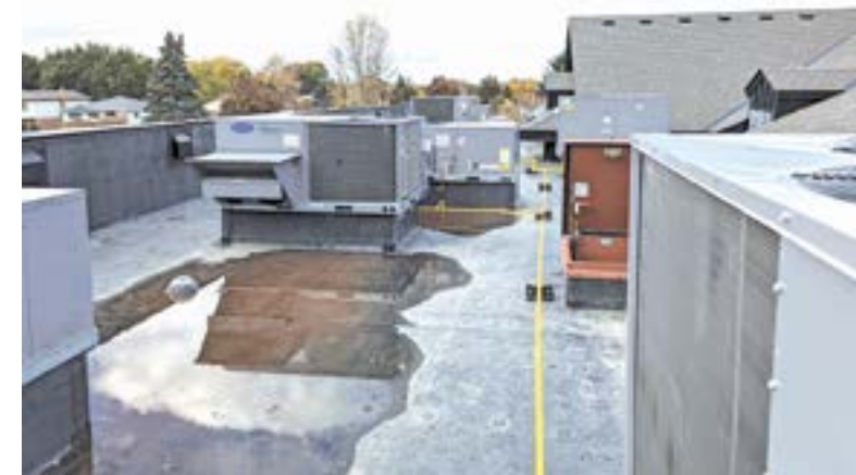
HVAC system for the new church is designed with the care of people in mind: All Saint's, Waterloo
